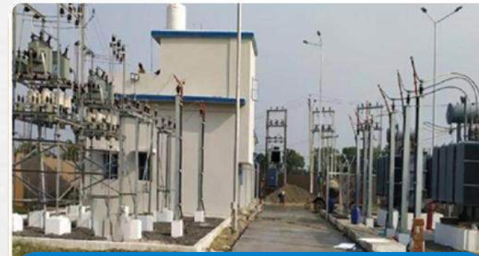
Rural Electrification Projects in Darbhanga and Muzaffarpur, Bihar, India
