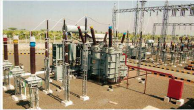
110/11 kV Substation at Koppal, Karnataka, India
