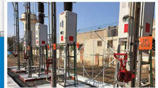
Overhead Railway Electrification under CORE Project
