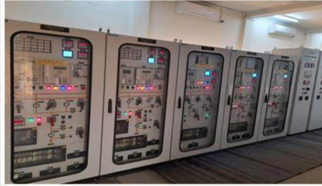
220/33 kV Substation at Amguri, Assam, India
