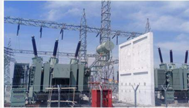
230/33 kV Substation at Thoothukudi District, Tamil Nadu, India
