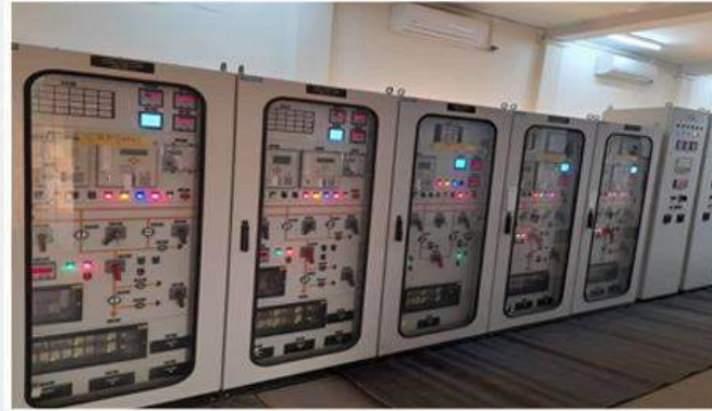
220/33 kV Substation at Amguri, Assam, India
