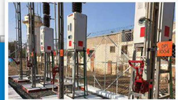
Overhead Railway Electrification under CORE Project
