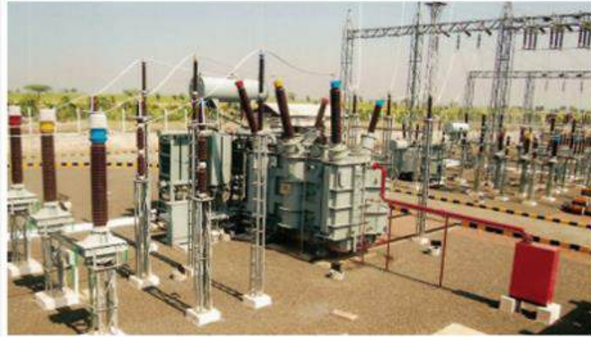
110/11 kV Substation at Koppal, Karnataka, India
