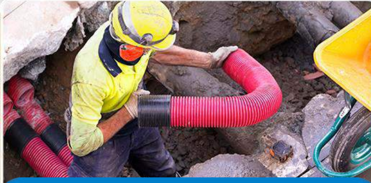
Strengthening Distribution Infrastructure in Tirupati & Vizag , Andhra Pradesh, India
